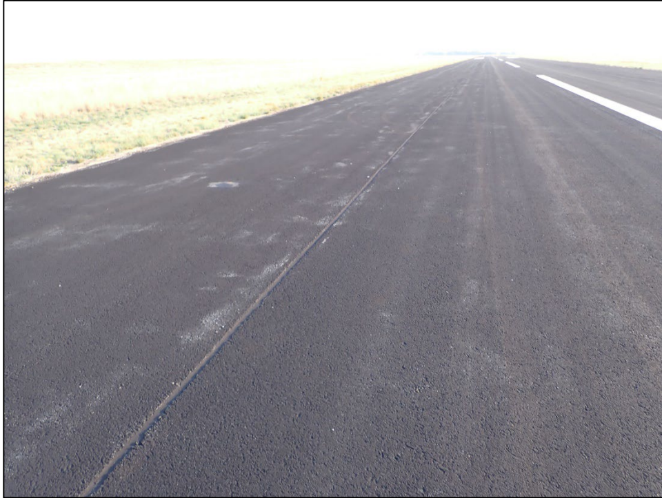
RW17-11-23: L&T Cracking
