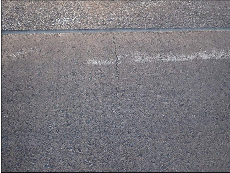
AP-02-04: L&T Cracking
