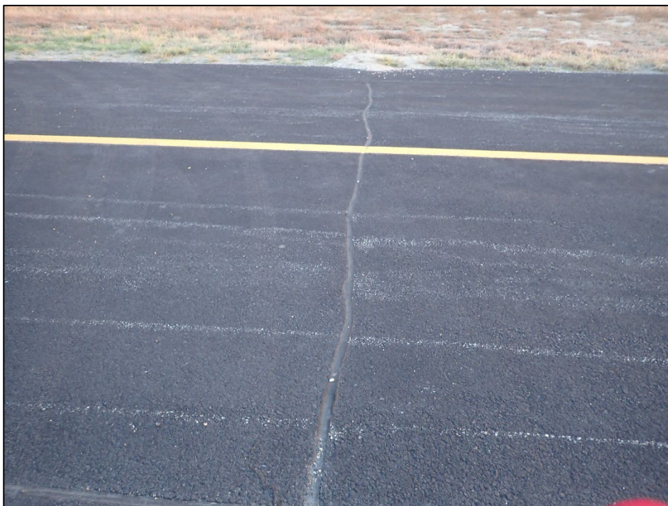
TW-12-03: L&T Cracking
