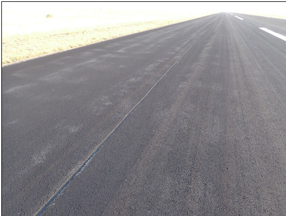
RW17-11-56: L&T Cracking
