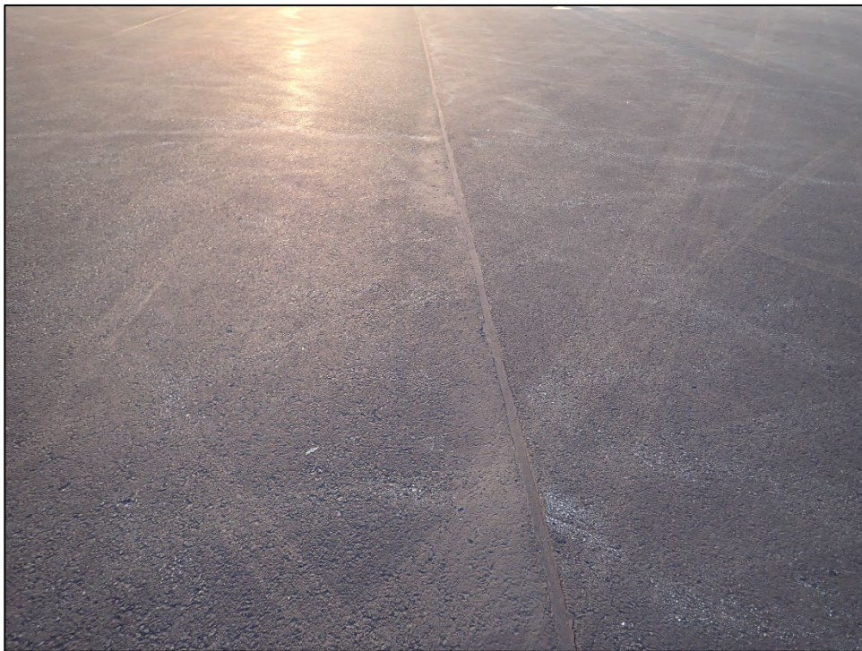
AP-11-01: L&T Cracking
